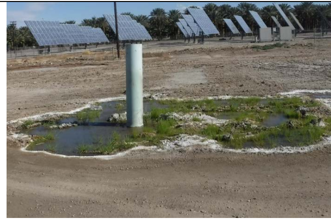
Image provided by CVWD prior to any repairs
