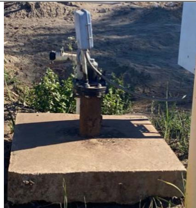
Image provided to CVWD of our finding. Well was repaired and no water leaking was found
