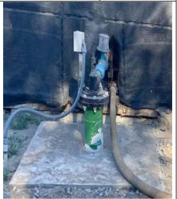
Image provided to CVWD of our finding. Well was repaired and no water leaking was found
